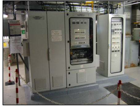
Figure 2, New Gaseous Sampling Cubicle
