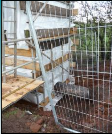
A two storey contamination control area is constructed to aid work at one of the break-in points north of the A75
